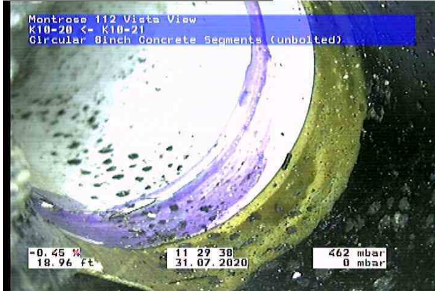
1896_59569f71-69b0-44e1-9b2e-fc7d46623be0_20200731_113503_786.jpg, 00:01:36, 17.92ft Tap Break-In Intruding at 10 o'clock, 4inch dim, 1inch intrusion, within 8 inch
