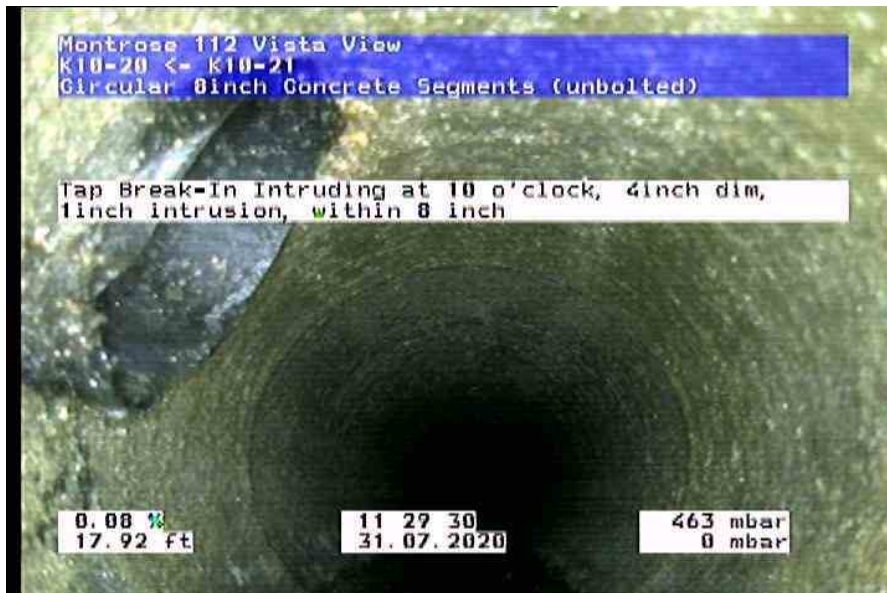
1896_f9fd0093-6589-4ab6-8125-7d4c5e019bdb_20200731_113455_152.jpg,00:01:36,17.92ft Tap Break-In Intruding at 10 o'clock, 4inch dim, 1inch intrusion, within 8 inch
