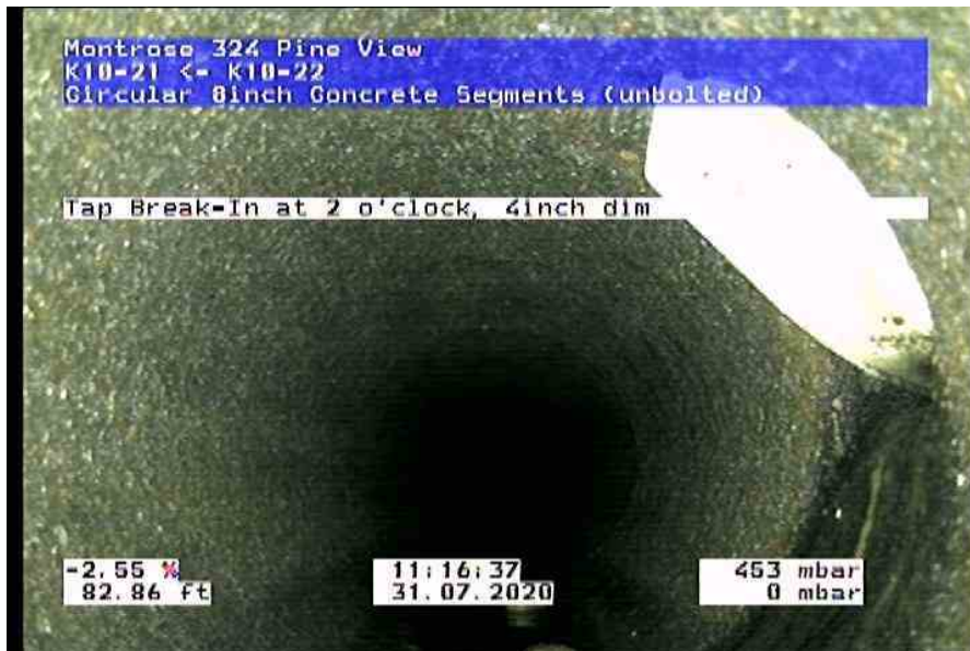
1755_db88b52a-e615-4c85-bfd9-ecc9aa972c8f_20200731_112202_541.jpg, 00:04:57, 82.86ft Tap Break-In at 2 o'clock, 4inch dim
