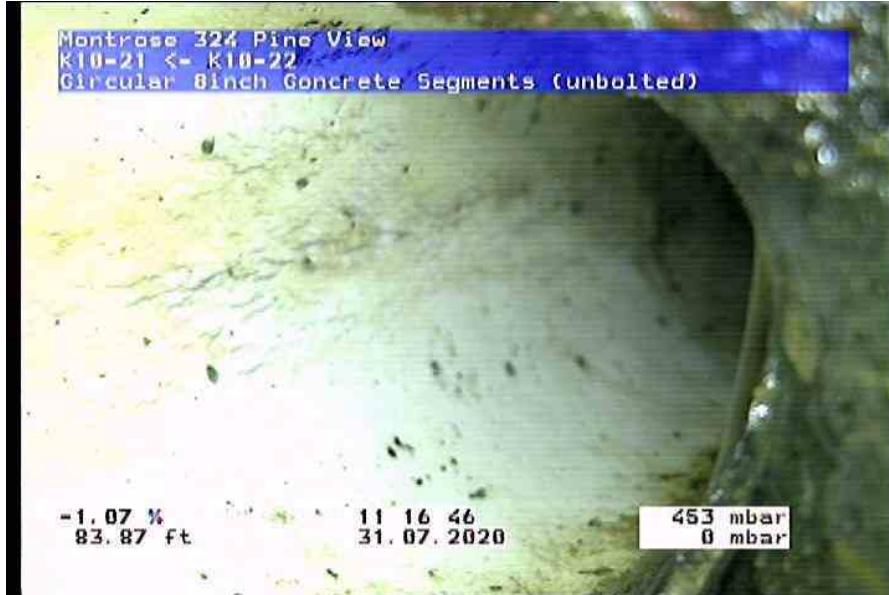
1755_bd561e51-e4de-42af-9349-f0d39c8823c1_20200731_112211_594.jpg, 00:04:57, 82.86ft Tap Break-In at 2 o'clock, 4inch dim
