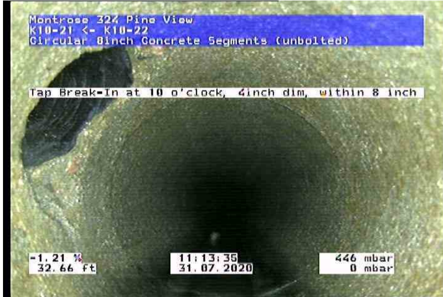
1755_5f2f19fc-ea83-495b-bdfa-cbcb9377fd16_20200731_111901_048.jpg, 00:01:54, 32.66ft Tap Break-In at 10 o'clock, 4inch dim, within 8 inch
