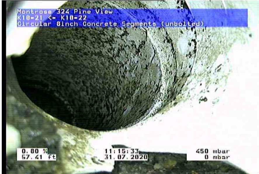
1755_0dea2bb6-0d05-4922-bf21-cfda75943ab7_20200731_112058_981.jpg, 00:03:47, 56.50ft Tap Break-In Intruding at 10 o'clock, 4inch dim, 1inch intrusion, within 8 inch
