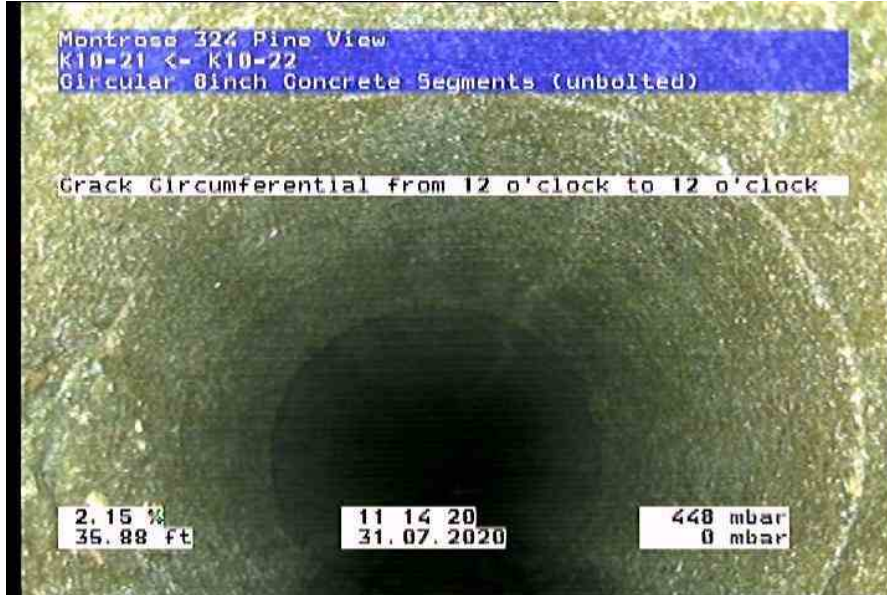
1755_7d7d11e3-55e3-495b-8616-e3906de18084_20200731_111945_875.jpg, 00:02:41, 35.88ft Crack Circumferential from 12 o'clock to 12 o'clock
