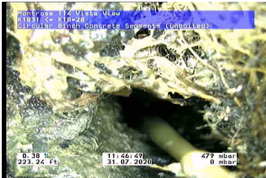
1740_dc919156-5063-46a6-aa2f-73c7b2333f3f_20200731_115214_428.jpg, 00:11:09, 222.95ft Tap Break-In Defective at 10 o'clock, 4inch dim
