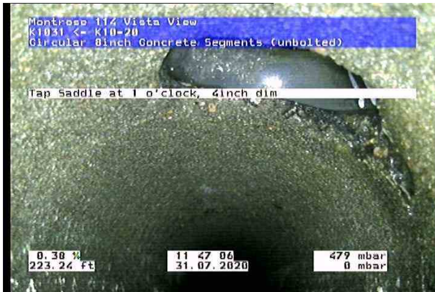
1740_daf8c50f-a101-4076-9400-631a685e8c60_20200731_115231_911.jpg, 00:11:54, 223.24ft Tap Saddle at 1 o'clock, 4inch dim
