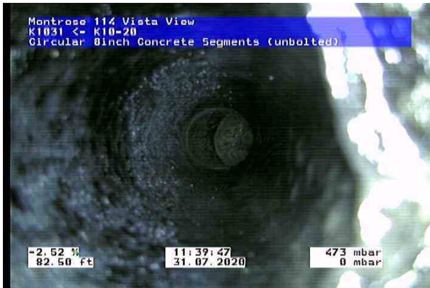
1740_e2bdc80e-12e1-40f8-a828-a293ef7a5154_20200731_114512_394.jpg, 00:04:28, 81.54ft Tap Break-In at 2 o'clock, 4inch dim, within 8 inch
