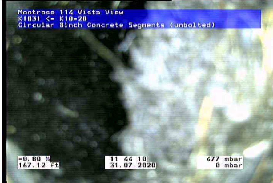
1740_3f4a5f8d-6ae9-4816-bcb0-356b424b5023_20200731_114935_939.jpg, 00:08:33, 165.89ft Tap Break-In Defective at 3 o'clock, 4inch dim
