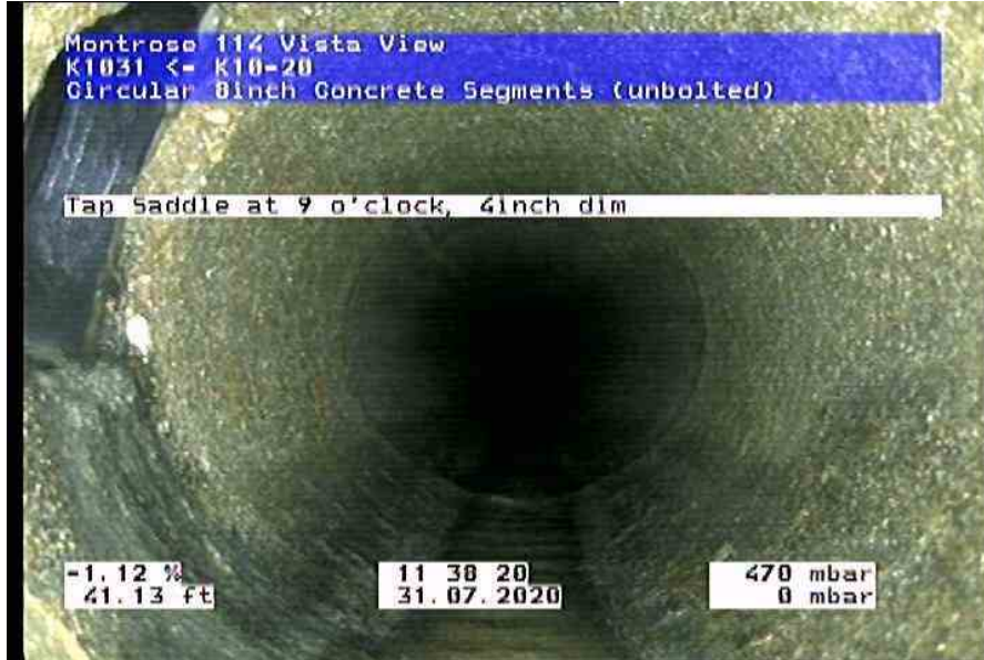
1740_aafdc0de-a642-4c30-a2cb-bb815c6b9358_20200731_114345_398.jpg,00:03:08,41.13ft Tap Saddle at 9 o'clock, 4inch dim
