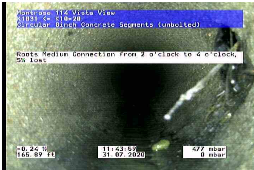
1740_50303b2d-e142-4060-966d-4505c76047c1_20200731_114924_424.jpg, 00:08:47, 165.89ft Roots Medium Connection from 2 o'clock to 4 o'clock, 5% lost
