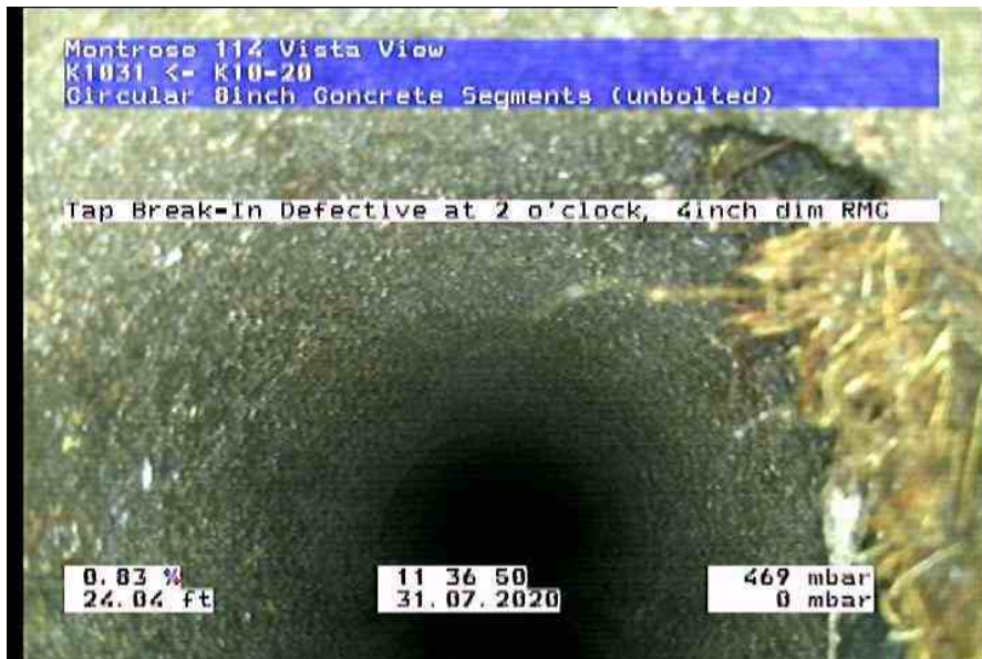
1740_400529b0-4bd0-4ec7-acd2-d002d2e4ddae_20200731_114215_191.jpg, 00:01:38, 24.04ft Tap Break-In Defective at 2 o'clock, 4inch dim
