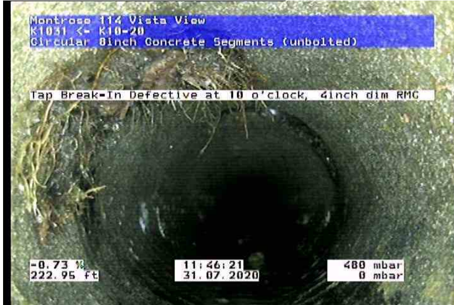
1740_e6c8afd0-1eb7-4964-936e-167ff9fbae09_20200731_115146_314.jpg, 00:11:09, 222.95ft Tap Break-In Defective at 10 o'clock, 4inch dim
