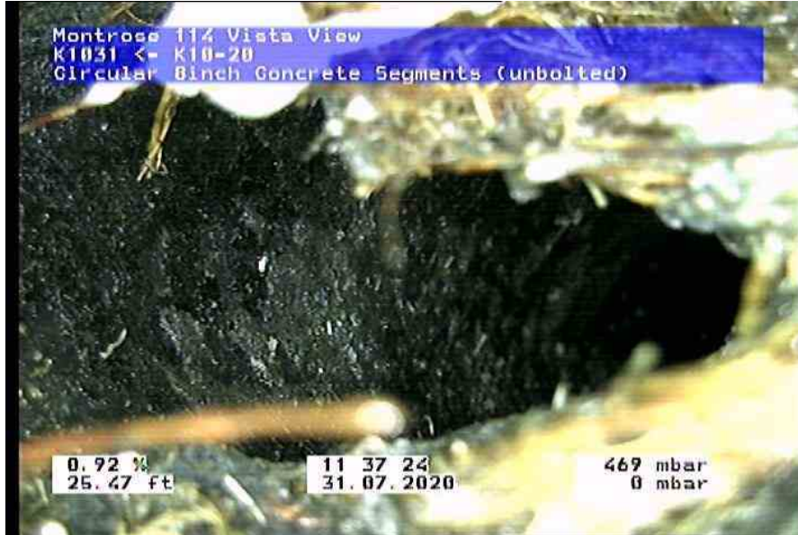
1740_b090610c-e417-44db-9cde-c99883c57729_20200731_114249_747.jpg, 00:01:38, 24.04ft Tap Break-In Defective at 2 o'clock, 4inch dim
