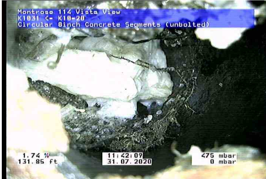
1740_808e9b22-5b71-4ce9-bee7-baaa419aa1be_20200731_114734_727.jpg, 00:06:20, 130.82ft Tap Break-In Defective at 10 o'clock, 4inch dim
