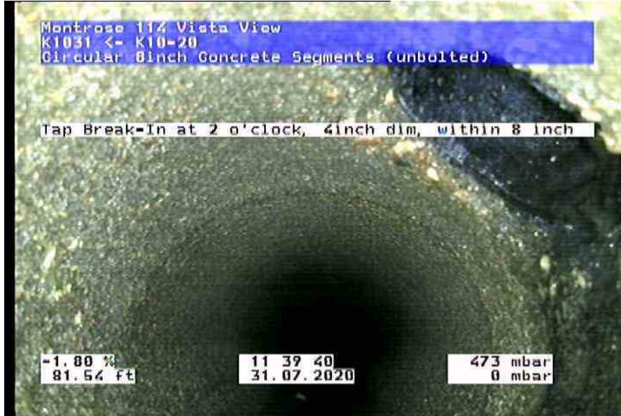
1740_99538d55-1a2f-48fc-8950-f86a0d856b6f_20200731_114505_636.jpg, 00:04:28, 81.54ft Tap Break-In at 2 o'clock, 4inch dim, within 8 inch
