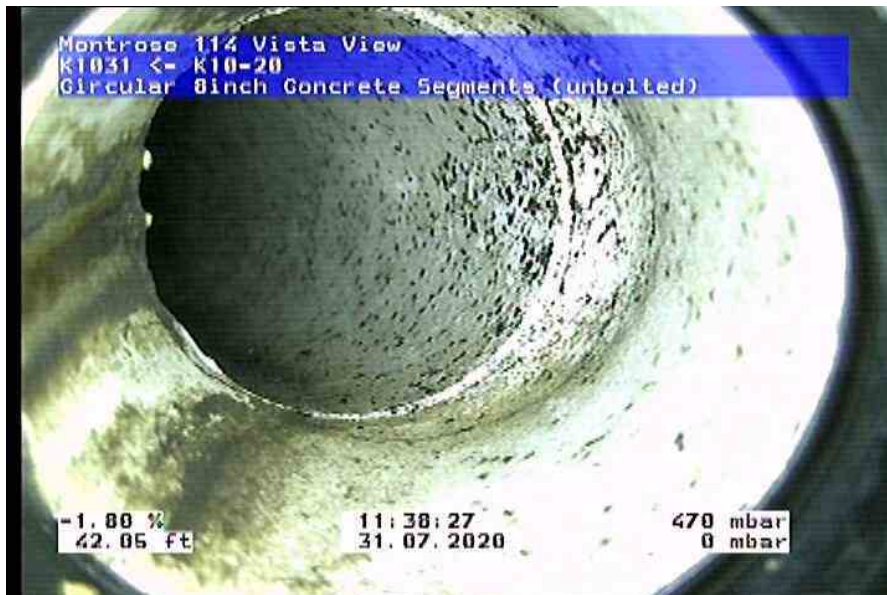
1740_bdb178ae-7157-486d-b695-3cc774091856_20200731_114352_318.jpg,00:03:08,41.13ft Tap Saddle at 9 o'clock, 4inch dim
