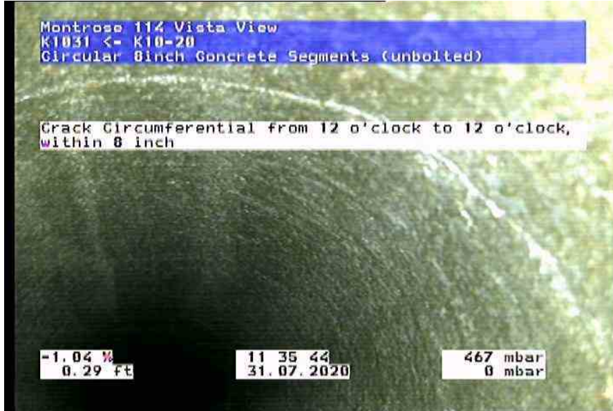
1740_57650a6e-aed2-4519-8570-5ae3f6a75886_20200731_114109_591.jpg, 00:00:32, 0.29ft Crack Circumferential from 12 o'clock to 12 o'clock, within 8 inch
