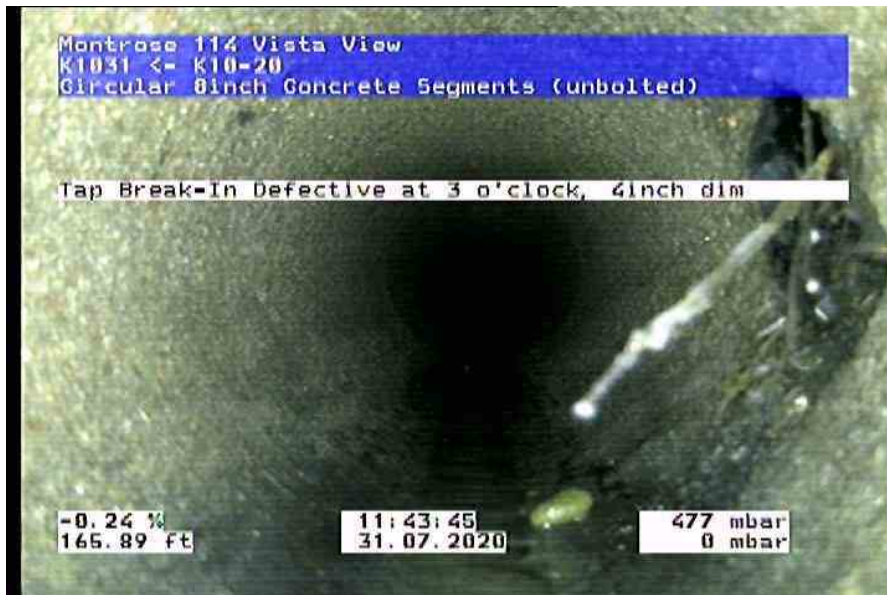
1740_91869521-bbe6-4073-b03d-7585c0b0f748_20200731_114910_934.jpg, 00:08:33, 165.89ft Tap Break-In Defective at 3 o'clock, 4inch dim
