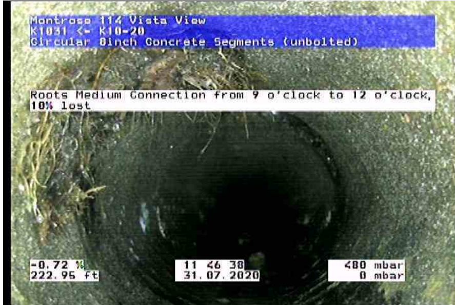
1740_27860731-f72f-46f4-9e8a-c8545b8c2357_20200731_115203_925.jpg, 00:11:26, 222.95ft Roots Medium Connection from 9 o'clock to 12 o'clock, 10% lost
