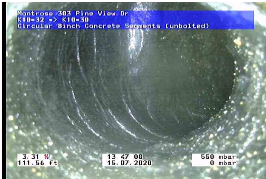
2228_19d856d2-ffb4-4093-a5b3-7435951c7bca_20200715_135232_814.jpg, 00:16:37, 110.41ft Tap Break-In at 2 o'clock, 4inch dim
