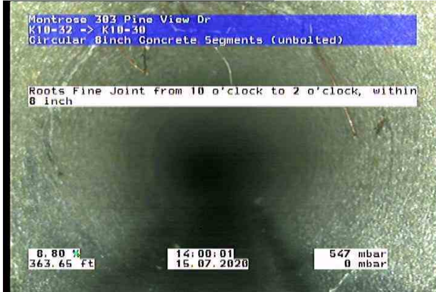
2228_9a07a94a-6273-426a-a1f7-0255191898c6_20200715_140525_848.jpg, 00:29:49, 363.65ft Roots Fine Joint from 10 o'clock to 2 o'clock, within 8 inch
