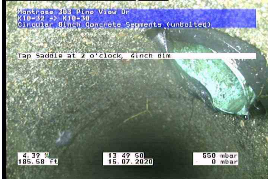
2228_dbf51b7f-7b05-4133-9008-7e1feaa3a52f_20200715_135514_267.jpg, 00:19:38, 185.58ft Tap Saddle at 2 o'clock, 4inch dim
