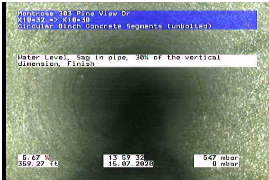
2228_2be6c9c7-9d32-4617-8c23-442fe37856e7_20200715_140457_288.jpg, 00:29:21, 359.27ft Water Level, Sag in pipe, 30% of the vertical dimension, Finish
