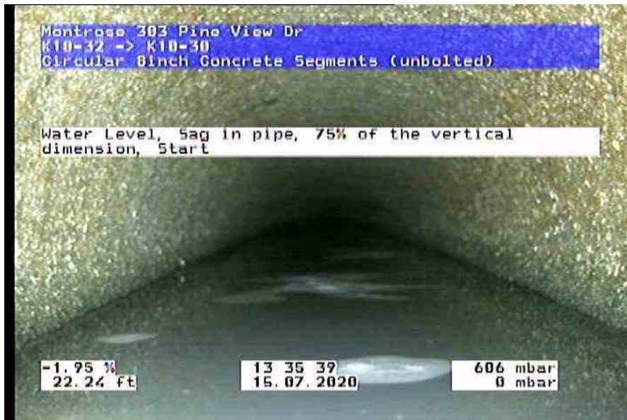
2228_04a1fd56-3379-4f69-ac94-100553f8bd91_20200715_134103_267.jpg, 00:05:27, 22.24ft Water Level, Sag in pipe, 75% of the vertical dimension, Start
