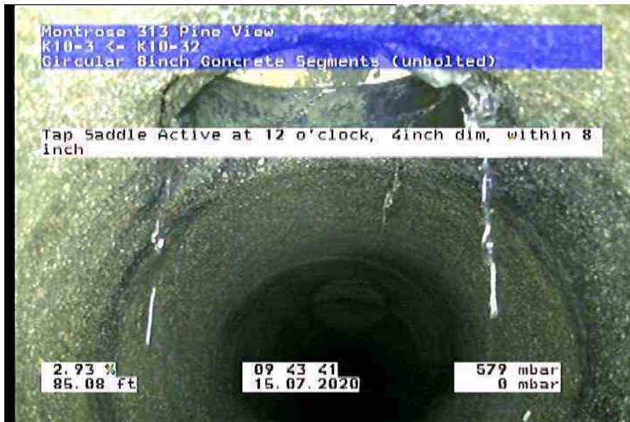
1843_c95d6925-9ad6-4c5a-9e48-1c2307ec5223_20200715_094905_596.jpg, 00:09:25, 85.08ft Tap Saddle Active at 12 o'clock, 4inch dim, within 8 inch
