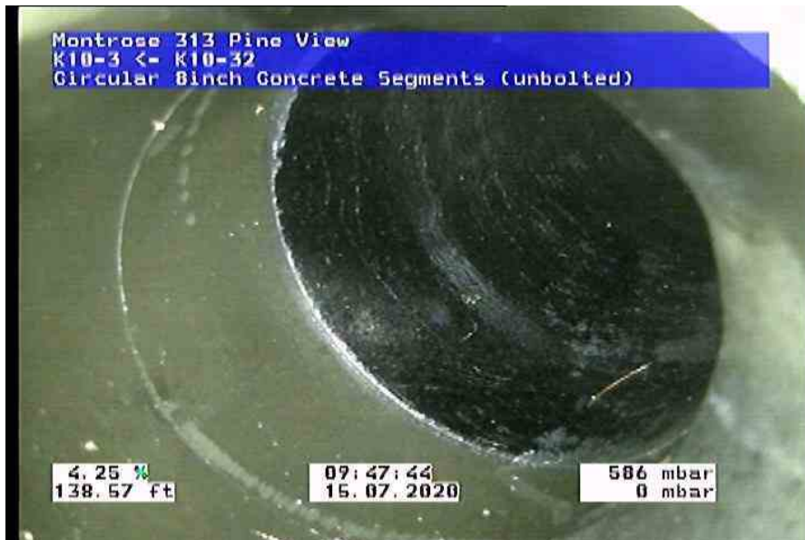
1843_1d5c3e9c-7aba-4272-aa50-c52371ee656e_20200715_095308_997.jpg, 00:12:37, 136.99ft Tap Saddle at 2 o'clock, 4inch dim
