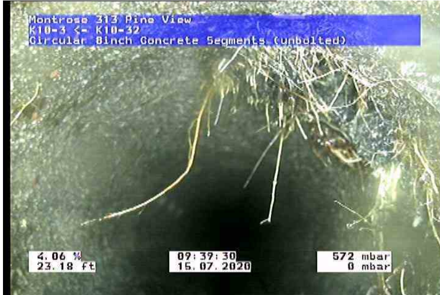
1843_9a42bb62-9566-4822-b6a5-bb8ed23d547d_20200715_094454_470.jpg, 00:04:37, 23.18ft Tap Break-In Defective at 2 o'clock, 4inch dim
