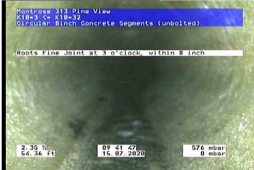
1843_242a7481-1aec-449f-935f-1e9734170bac_20200715_094712_201.jpg, 00:07:32, 54.36ft Roots Fine Joint at 3 o'clock, within 8 inch
