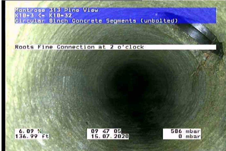
1843_e8323419-8eb3-40a8-bbd8-aa6301419261_20200715_095229_764.jpg, 00:12:50, 136.99ft Roots Fine Connection at 2 o'clock
