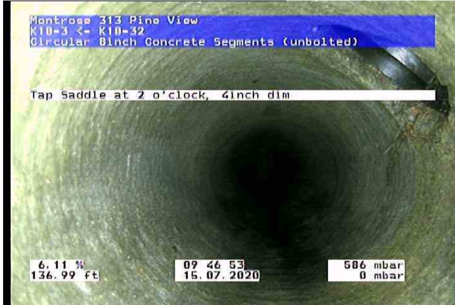
1843_97c3694a-8b59-419c-81d9-3efe309963b3_20200715_095217_504.jpg, 00:12:37, 136.99ft Tap Saddle at 2 o'clock, 4inch dim
