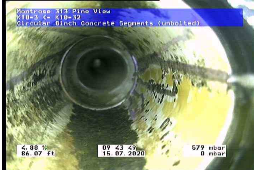
1843_d406e683-6c12-4d23-8b24-3252ba16b479_20200715_094914_420.jpg, 00:09:25, 85.08ft Tap Saddle Active at 12 o'clock, 4inch dim, within 8 inch
