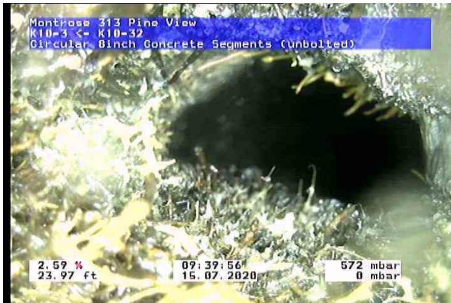
1843_5b901da6-cb23-41a4-b9b4-69754cc50892_20200715_094520_780.jpg, 00:04:37, 23.18ft Tap Break-In Defective at 2 o'clock, 4inch dim
