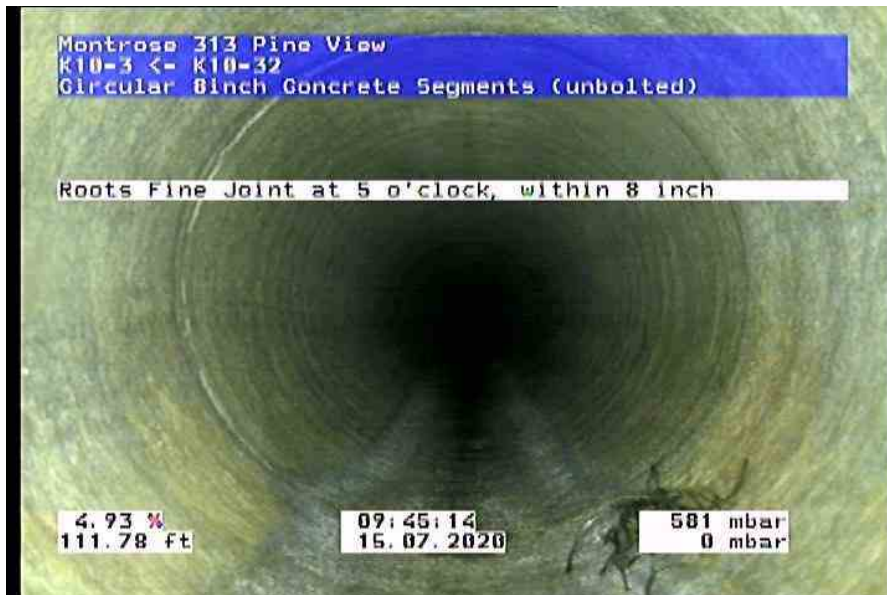
1843_50bb3915-6189-477e-a763-f1da52e855b5_20200715_095038_549.jpg, 00:10:58, 111.78ft Roots Fine Joint at 5 o'clock, within 8 inch
